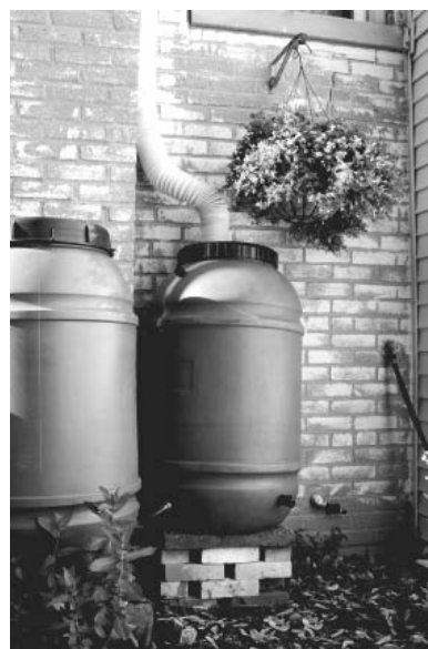
Linked rain barrels reap rainfall. Pilot rainwater harvesting programs have been started in LA and Long Beach.
